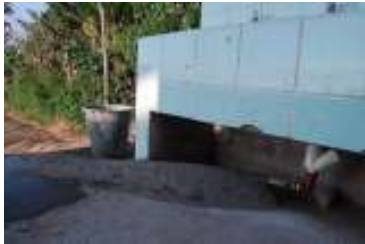
Fig 10. Diverted drainage from the hand washing station. Pipe is encased in concrete for protection.
