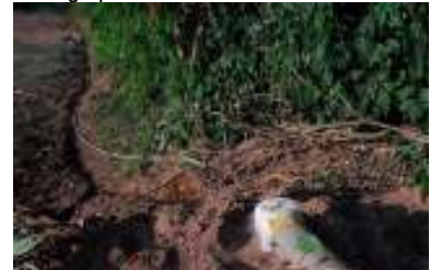
Fig 15. Water bottle is used as a reducer to send the septic tank effluent down a length of recycled water pipe, which follows the line of a trench.
