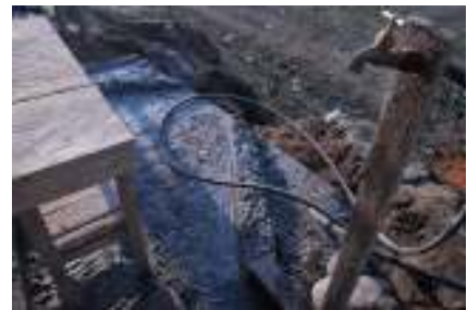
Fig 24. Finished base, on an incline with rainwater drainage channels. Temporary table for washing up in lieu of a sink. The drainage pipe that leads to the soakaway below is visible
