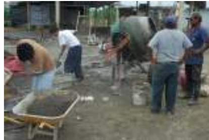
Fig 18. Minga, with assistance from the CoopEcuador labourers and machinery to mix the cement.
