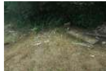
Fig 3: Septic tank. Note that the outflow runs down the bank onto the playing field
