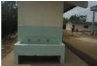
Fig 2: Hand washing station
