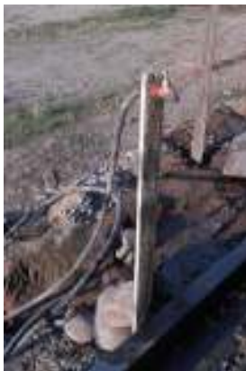
Fig 22. Temporary standpipe style tap, positioned above the rainwater drain.
